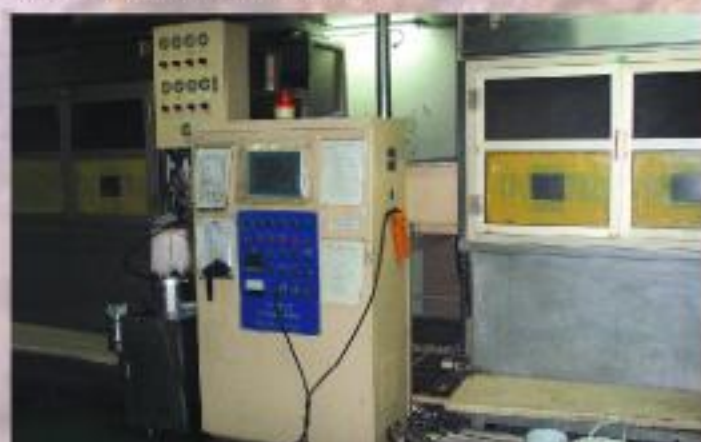
自動噴漆設備 AUTO-PAINTED EQUIPMENT
